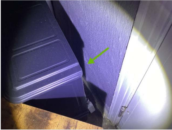
Rear wall efflorescence
